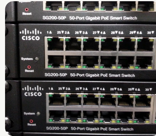
Switching Cisco PoE
