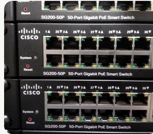
Cisco PoE switching
