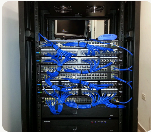
Structured cabling rack
