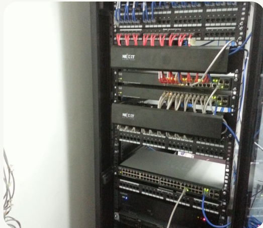
Installed equipment rack
