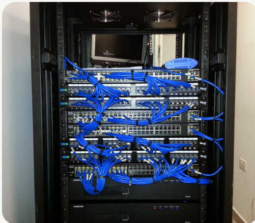
Structured cabling rack
