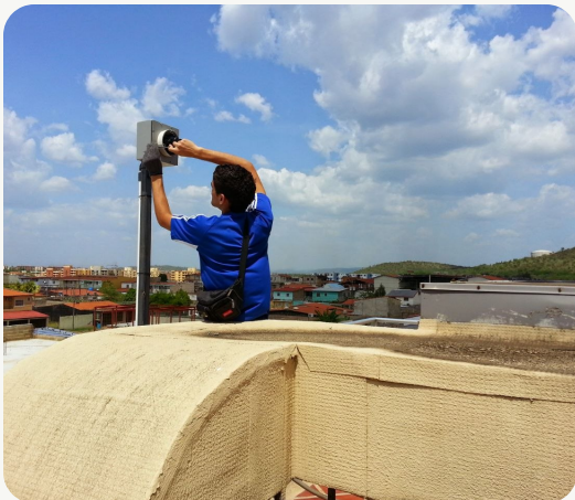
Exterior camera installation
